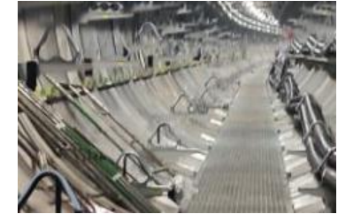
2022 China Smart Urban Utility Tunnel
