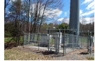
2022 Chile Smart Cell Tower
